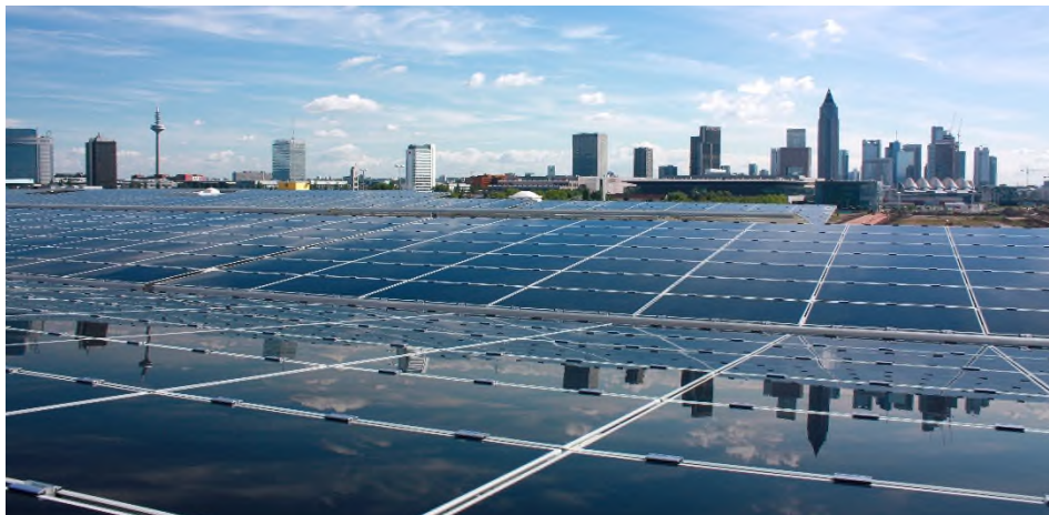
Solar panels on the Rebstock parking garage - one of Messe Frankfurt's three photovoltaic systems. Foto:
